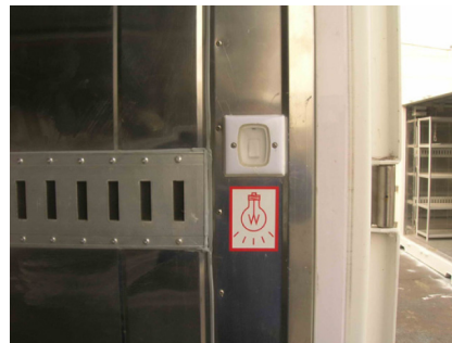
2 Light Switches on for each Compartment
